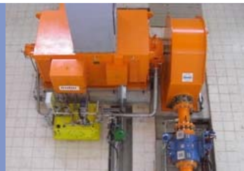
Turbine-generator unit after commissioning in December 2010
